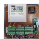
PCB, Power trans, Terminal block
